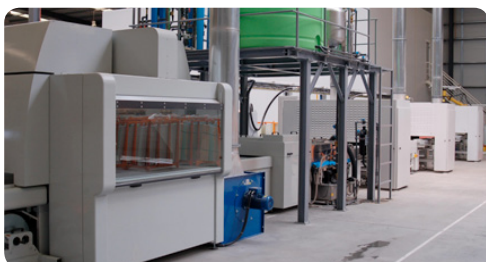
< Vindico PV+™ line in Portugal
